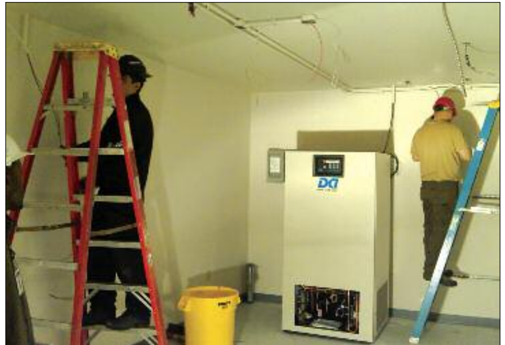
Richmond Redevelopment & Housing Authority Data Center
